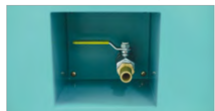
Spill drain port for clean internal management.
